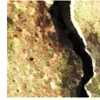
Figure 1: Original image of concrete crack.
